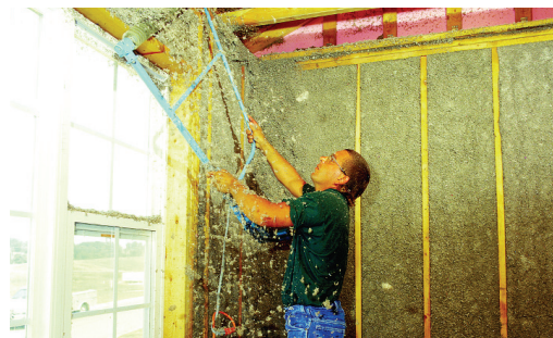
An installer “shaves” excess wet-spray cellulose fiber insulation from wall studs after it has dried.
